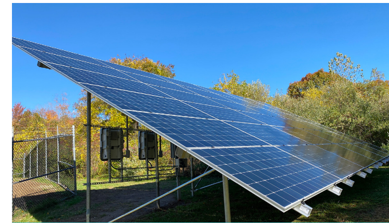
Colchester, CT – Connecticut Water completed the installation of solar panels at one of its smaller water systems which were sufficiently sized to fully meet energy requirements to pump, treat, and move water through the water system, effectively removing it from the power grid.
